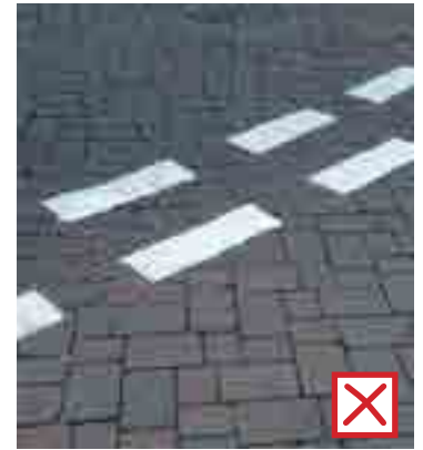
No block paving where white lining is required
