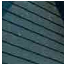
Black stained weatherboarding
