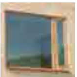
Timber natural stain
