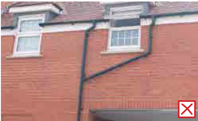
Rainwater goods will not diagonally cross the building elevation on any given street or edge.
