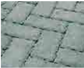
Permeable keyblock paving
