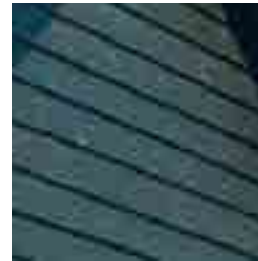
Black stained weatherboarding
